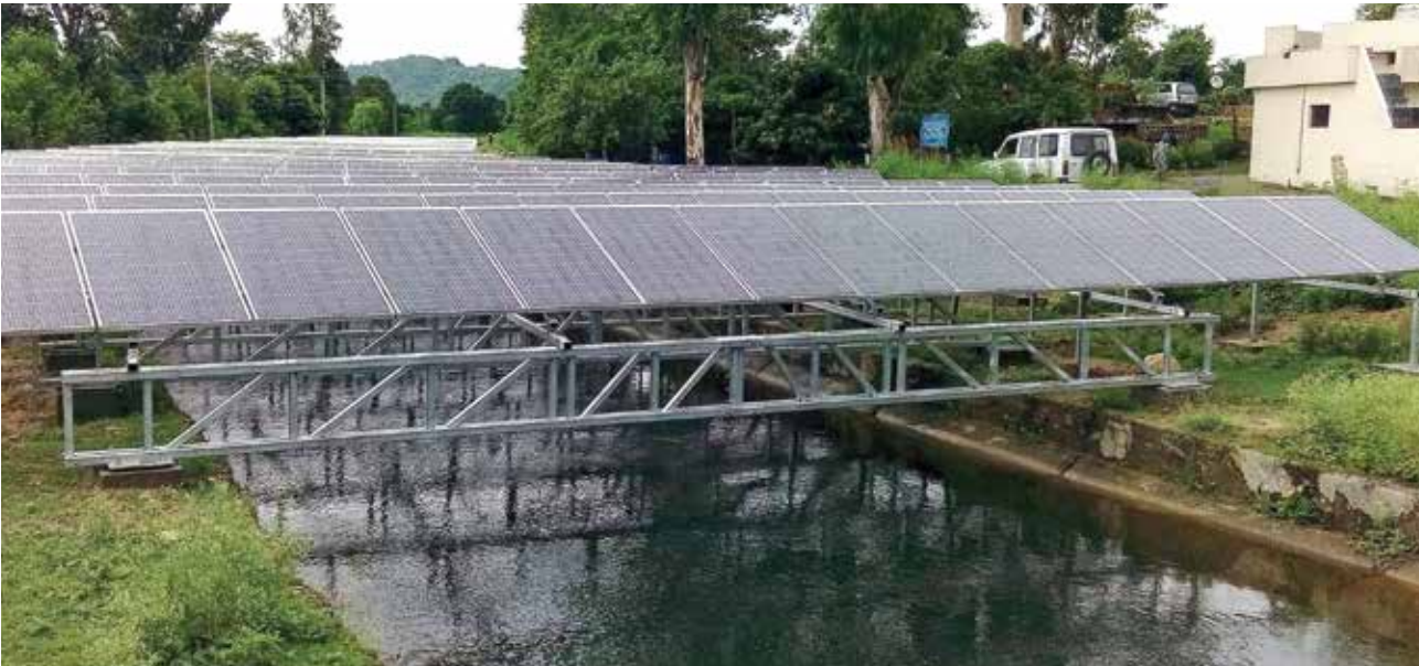
Canal Top Solar Power Plant for Lift Irrigation Pumping Station
