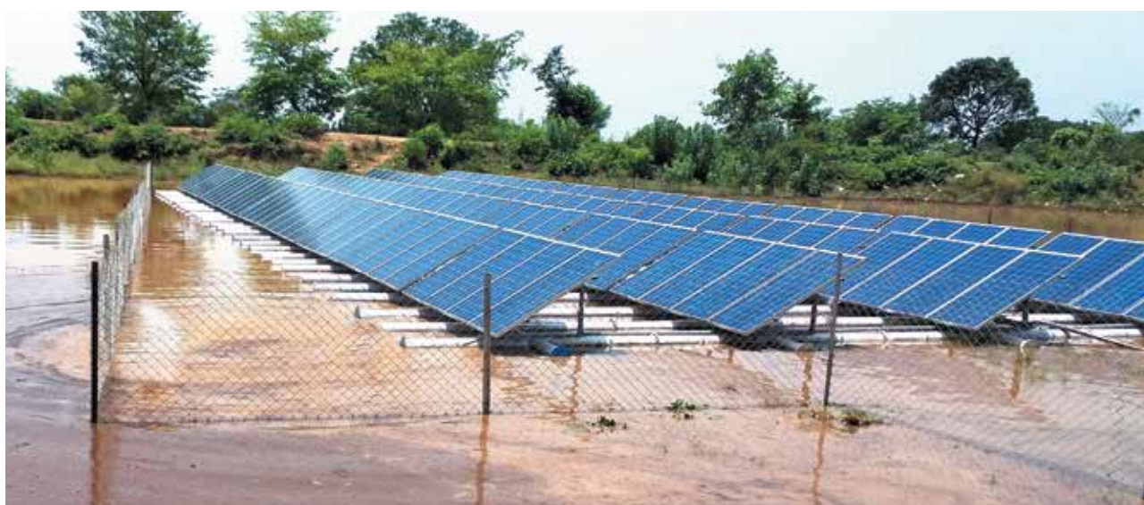
Jain Tarang (Floating) Platform in reservoir
