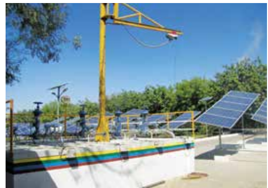
Surface pump testing
