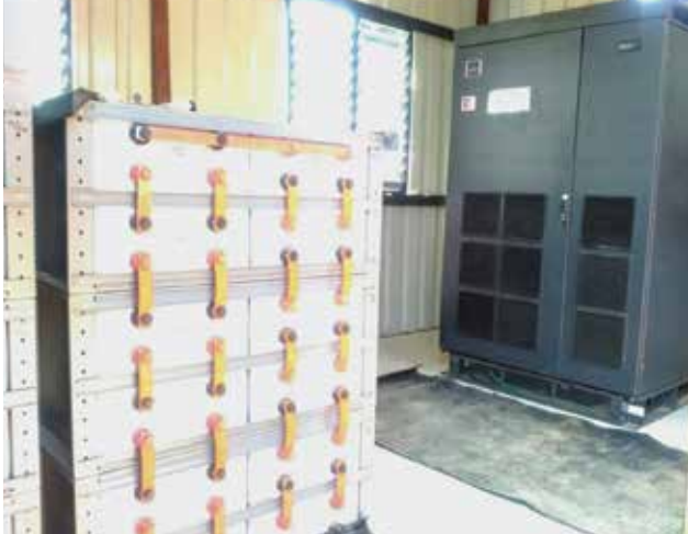
VRLA Battery Bank
