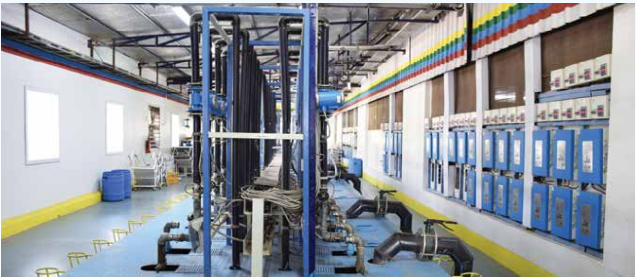
Jain Solar Pump Inplant Testing Center; Green Energy Park; Jain Valley, Jalgaon.
