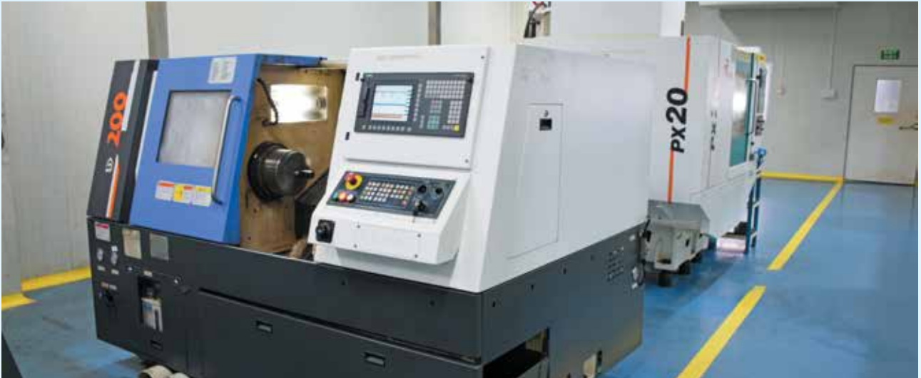
Jain Solar Pump Manufacturing Plant (Automatic CNC Machine) Green Energy Park; Jain Valley, Jalgaon.
