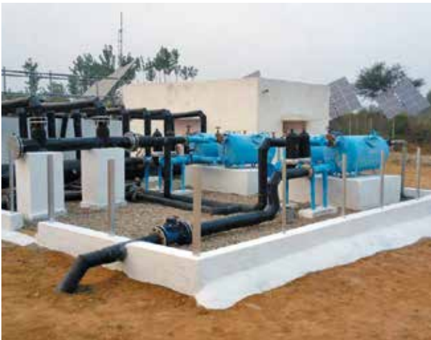
328 kW (245 hp) Solar Pumping Station
