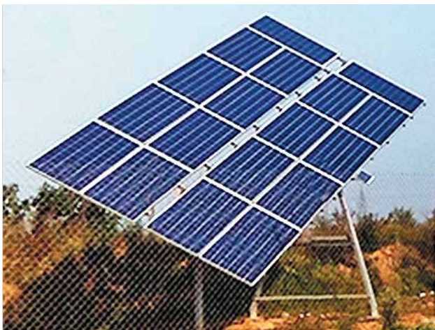
Single Axis Structure
