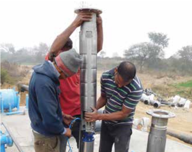
Solar Pump Assembly
