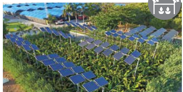
Solar AgroVoltaic Plant
