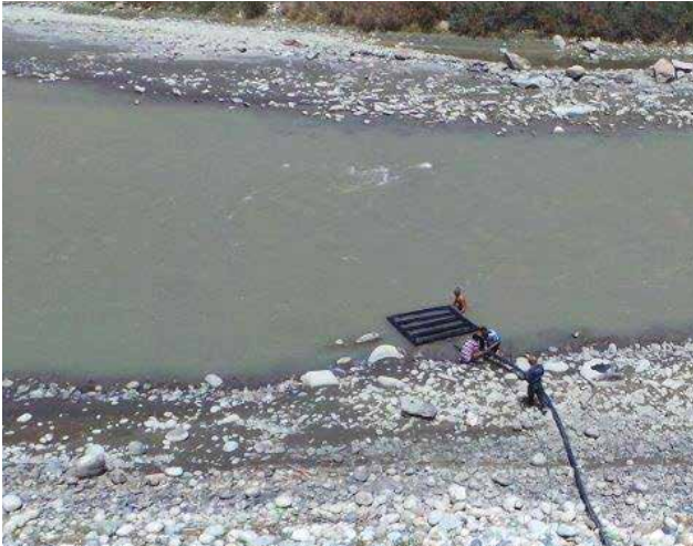
Floating Submersible Pump in Indus River
