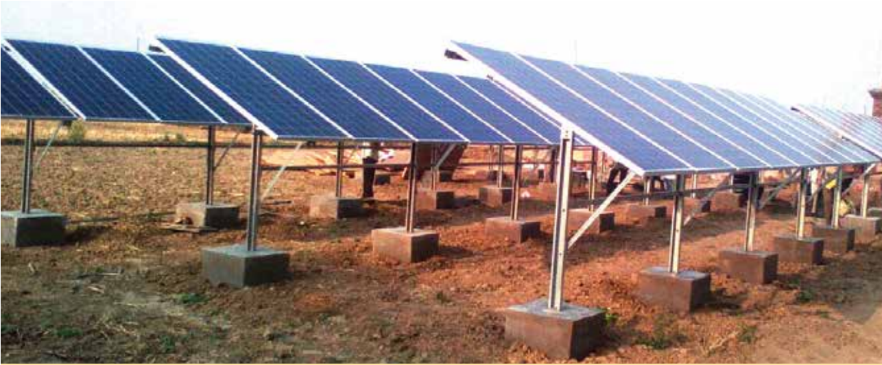
Fixed Type Solar Structure for Community Tube Wells
