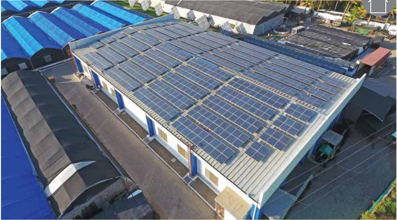
Solar Roof Top Grid Connected Plant
